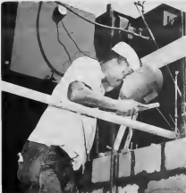
WELDING REINFORCING rods on a fire wall, above left, and building the fire wall between the two transformer is a part of the project, which will enable Lago to buy power from the government.
